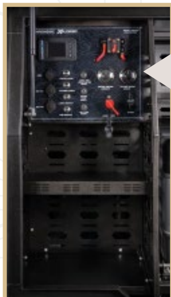
12V Control Panel
